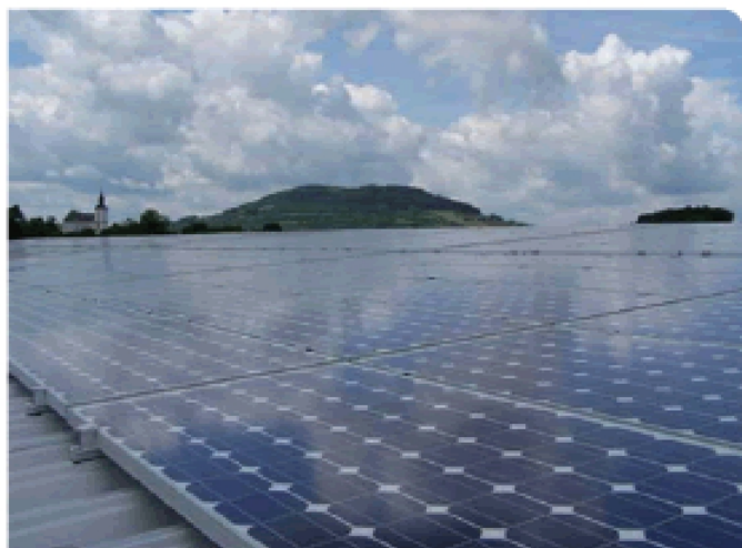
Agricultural roof PV plant
